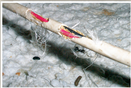
Gnawing on wires with droppings.*
