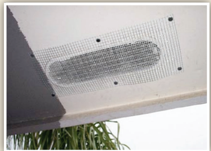
Soffit vent hole sealed with screen.*
