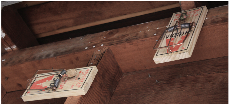
Proper trap placement on beams and rafters. Note rub marks on beams indicating rat trails.
